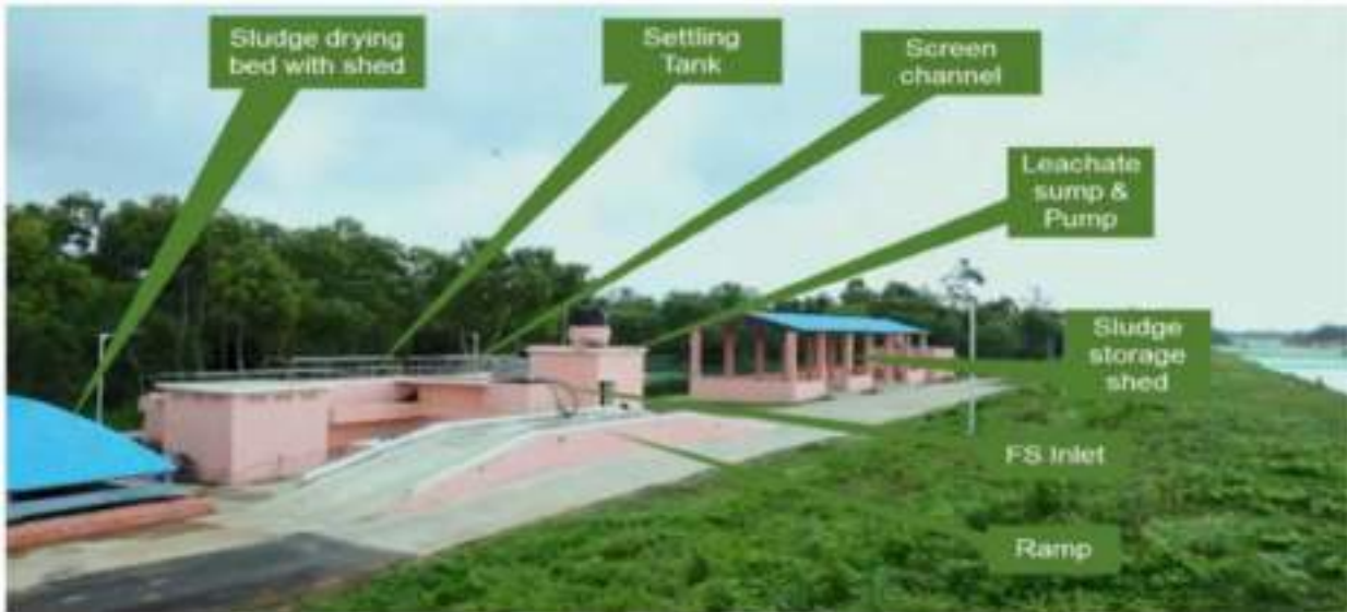
STP-cum-FSTP to treat sewage and faecal sludge in the same facility
